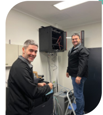
Focus Networks Server Upgrade Installation
