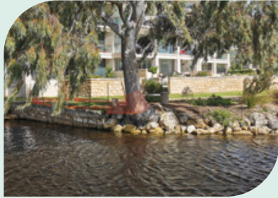
John Street riverwall repair, City of Fremantle. This project benefitted from Board funding for site investigations and detailed design in 2021-22, and implementation in 2022-23. Works to be completed in early 2024.
